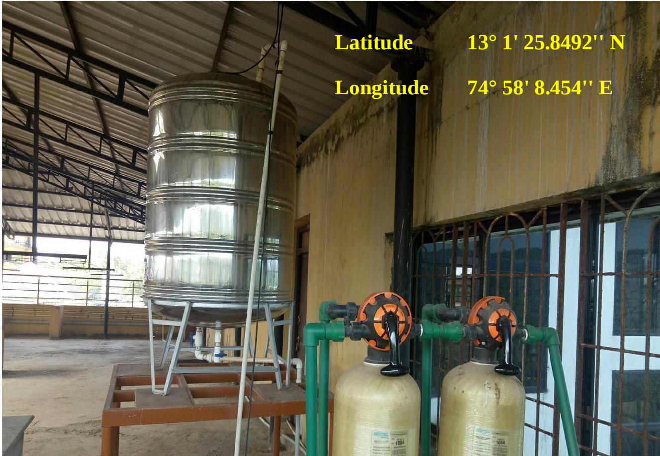
Solar Water Heater installed at Kaveri Ladies Hostel Block
